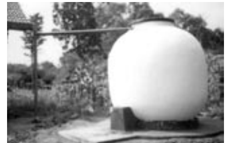
Aboveground rainwater harvesting tank
